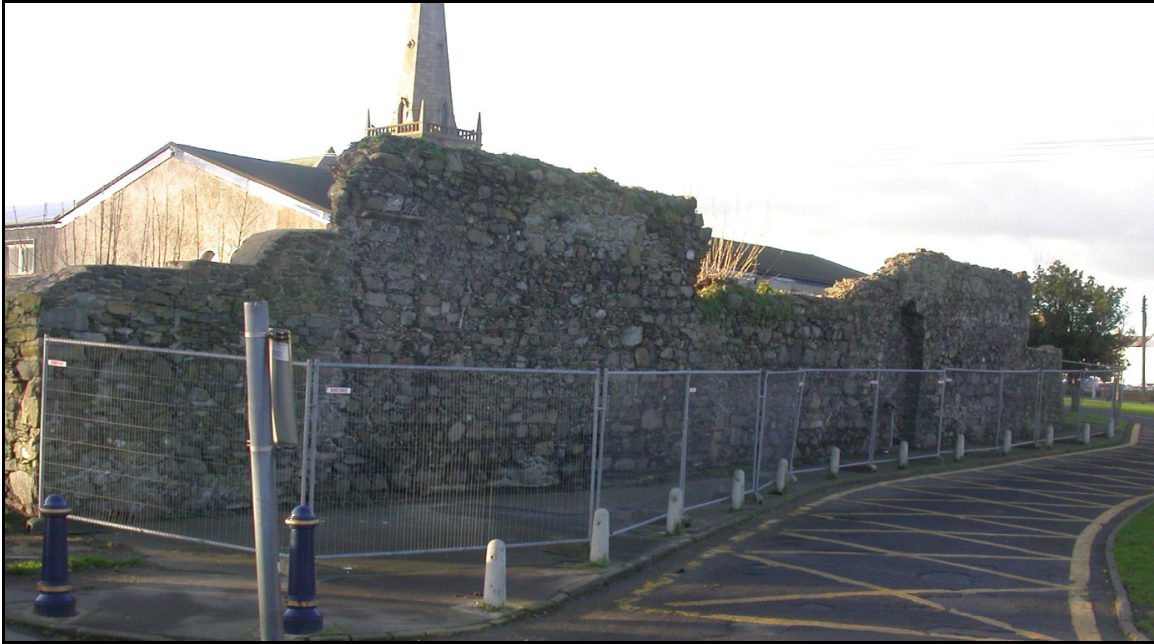
Plate 1: (Above) North face of Malachy's Wall (taken from north- east facing south-west).
