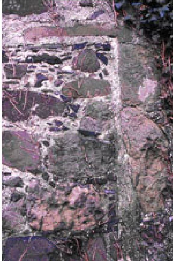
Plate Three: Part of a now infilled window, defined by neatly dressed stones, which survives on the north-facing side of Kilroot House.
