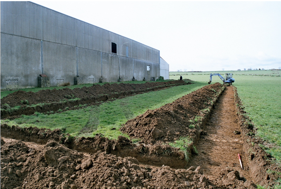
Plate 2: View of proposed development site from north-east after excavation of test trenches.
