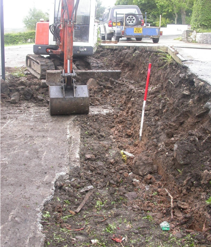
Plate 1: View of site from north after clearance and prior to excavation of foundation trench.
