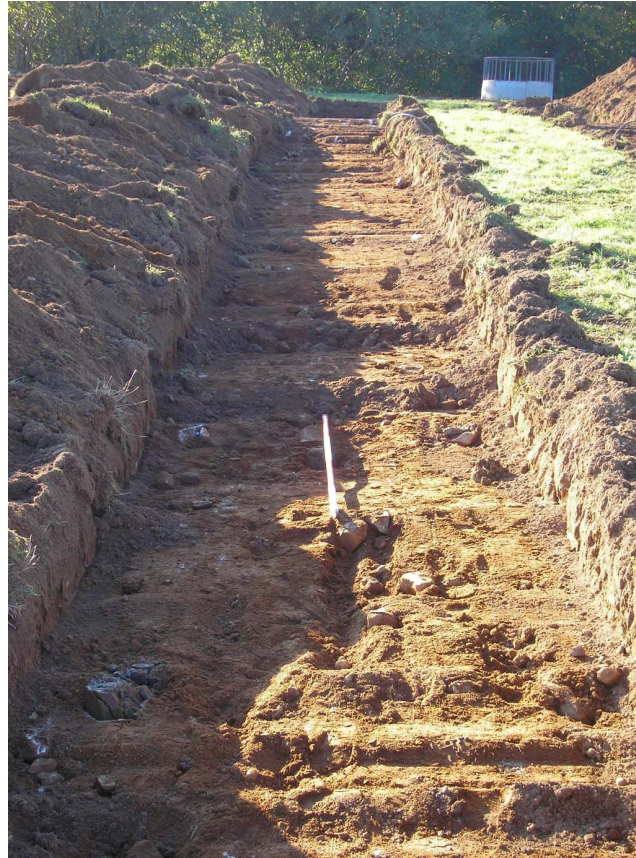
Plate Seven: Trench Four following excavation to subsoil (Context No. 403), looking west.
