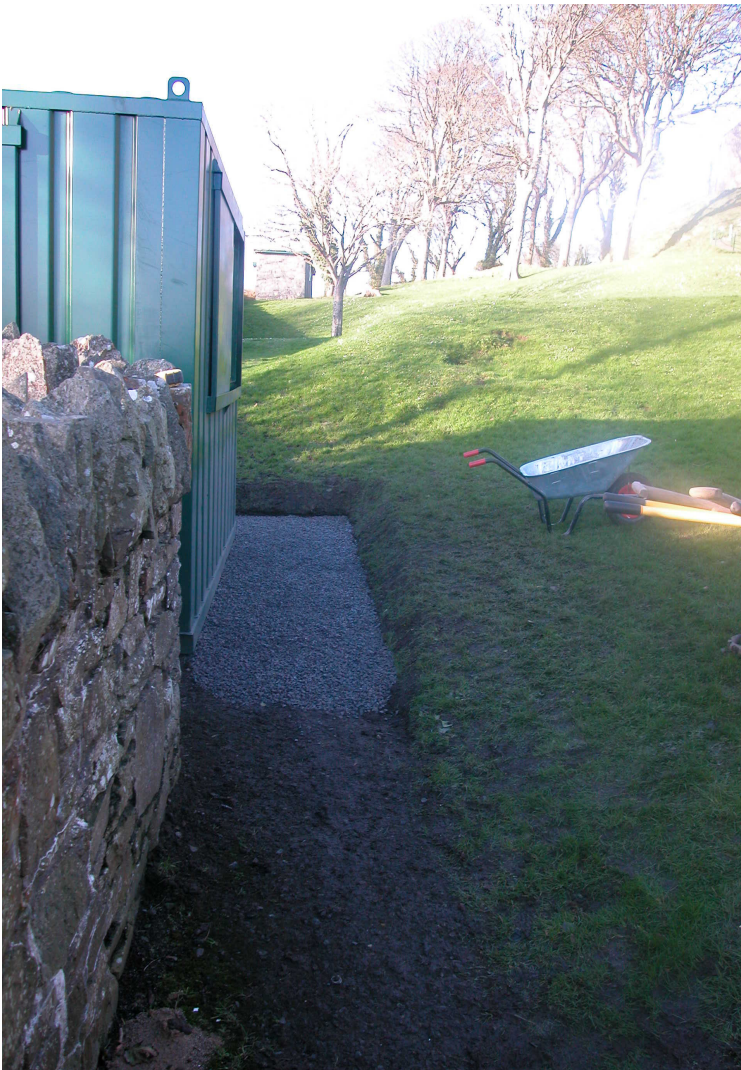
Plate 2: Trench 1 on north-east side of portacabin after excavation and laying of gravel.
