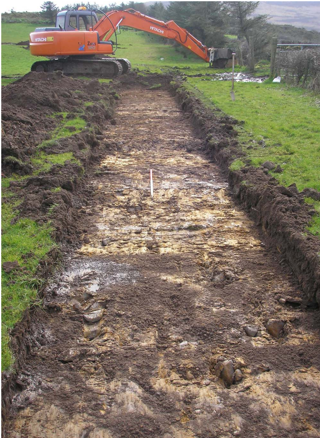
Plate 1: Trench One following excavation to subsoil (Context No. 104), looking south-east. NB surface water lying on the subsoil.
