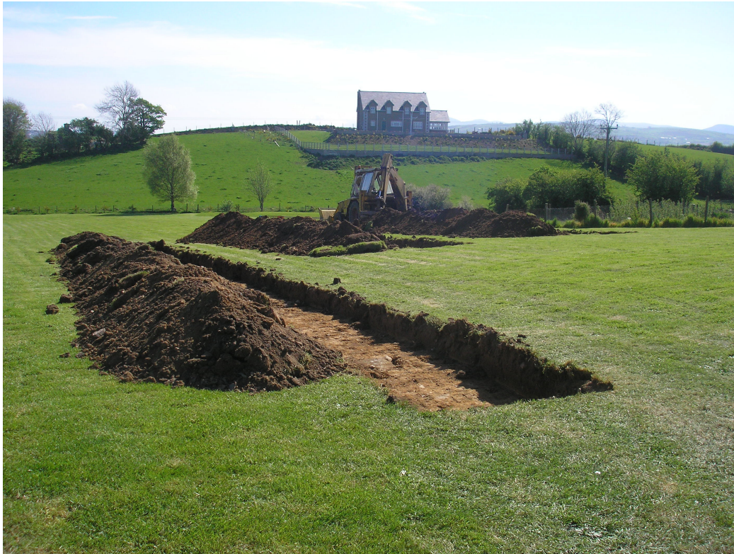
Plate Seven: General view of the application site following the excavation of the test trenches, looking south-east.
