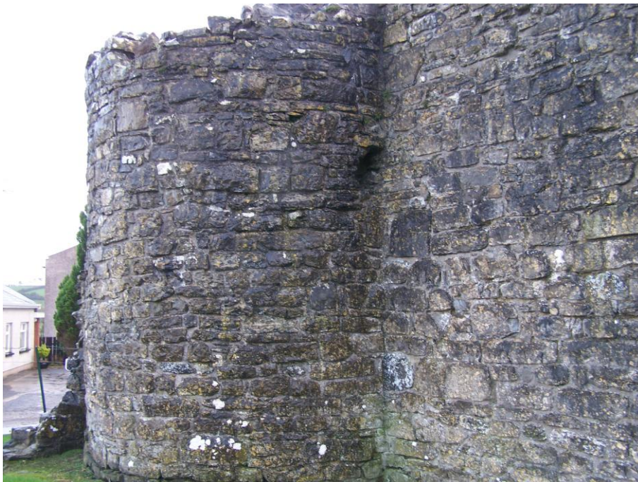
Plate 22: The circular flanker at the northern corner of the gatehouse, looking north-east
