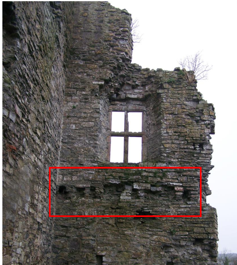
Plate 3: floor joist sockets below first floor window on south-western wall of main block (outlined in red), looking south-west
