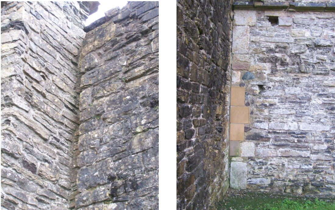
Plate 19 (left): The north-eastern junction between the castle and gatehouse walls, looking north-west, and Plate 20: The south-western junction between the castle and gatehouse walls, looking north-east
