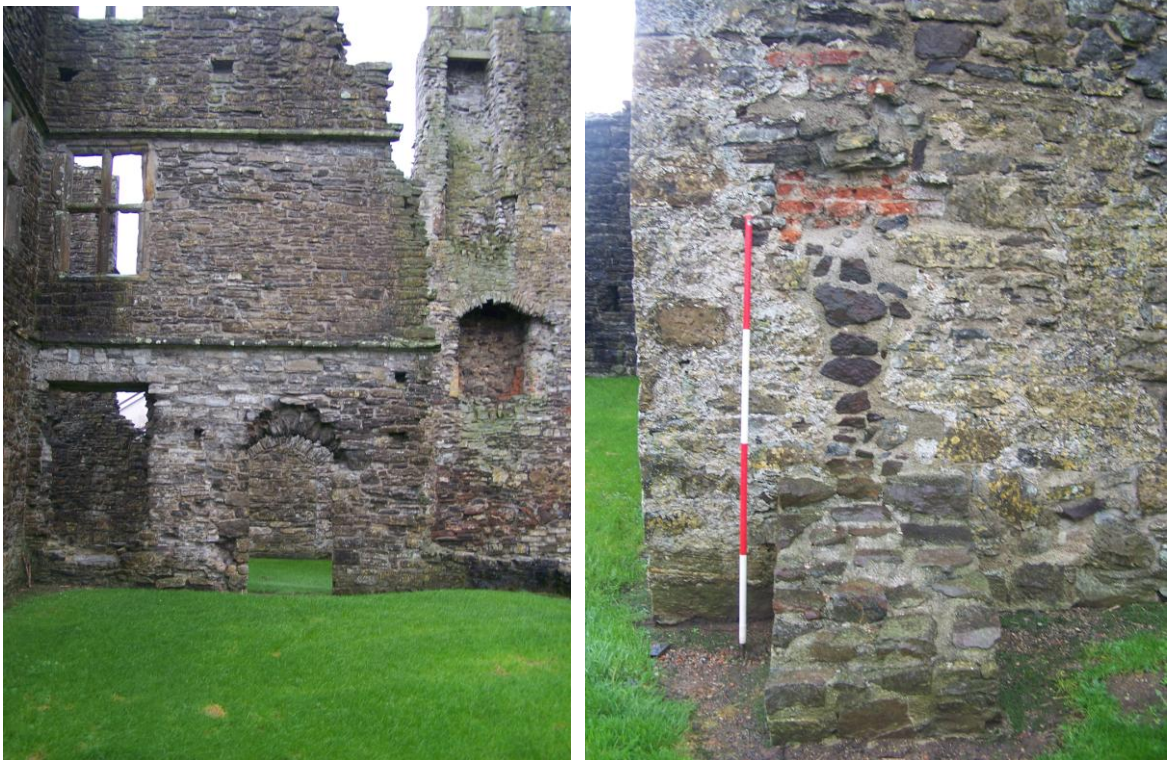
Plate 6 (left): The courtyard area between the two wings, looking south-east, and Plate 7: Traces of courtyard wall stump on the south-western wall of the north-eastern wing, looking north-east
