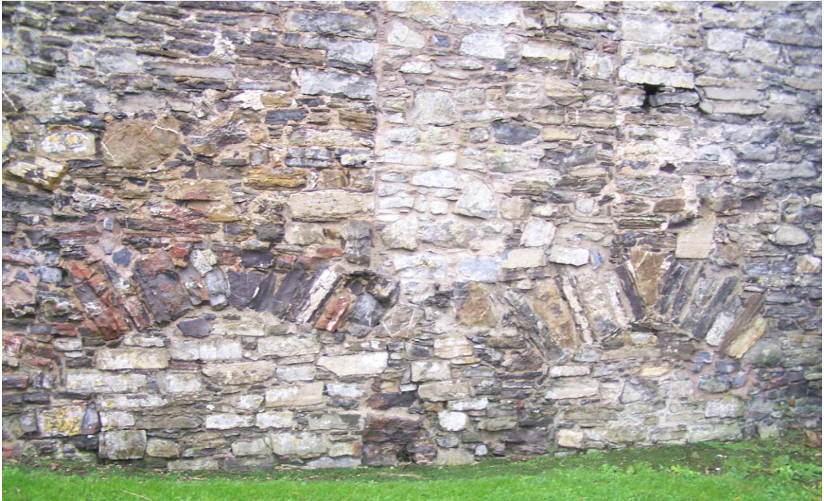
Plate 11: Blocked-up arches on the interior side of the south-eastern wall of the main block, looking south-east
