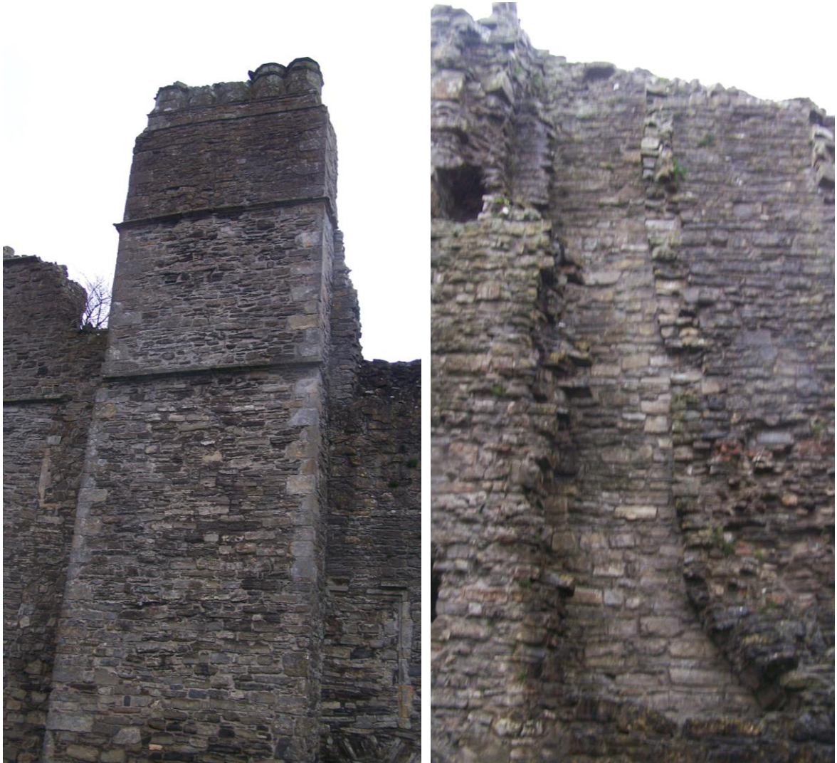
Plate 8 (left): Complete chimney stack on south-eastern façade of main block, looking north-west, and Plate 9: Interior of more northerly chimney stack on the south-eastern wall of the main block, looking south-east
