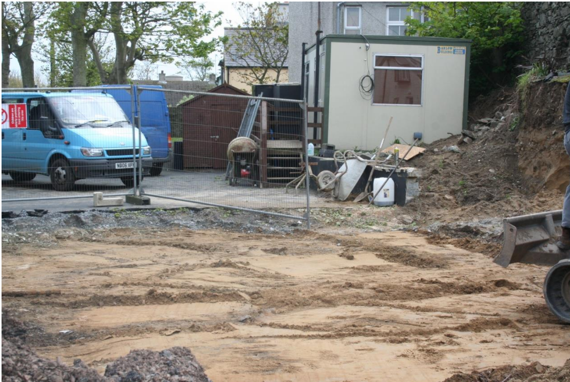
Plate 11: Tarmac driveway area on removal of tarmac and hardcore layer (C102), showing natural sand subsoil, looking south west.
