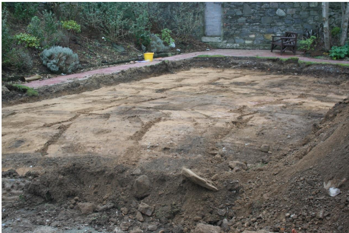
Plate 6: Garden area on the removal of contexts 101-104, showing natural sand subsoil, looking south east.
