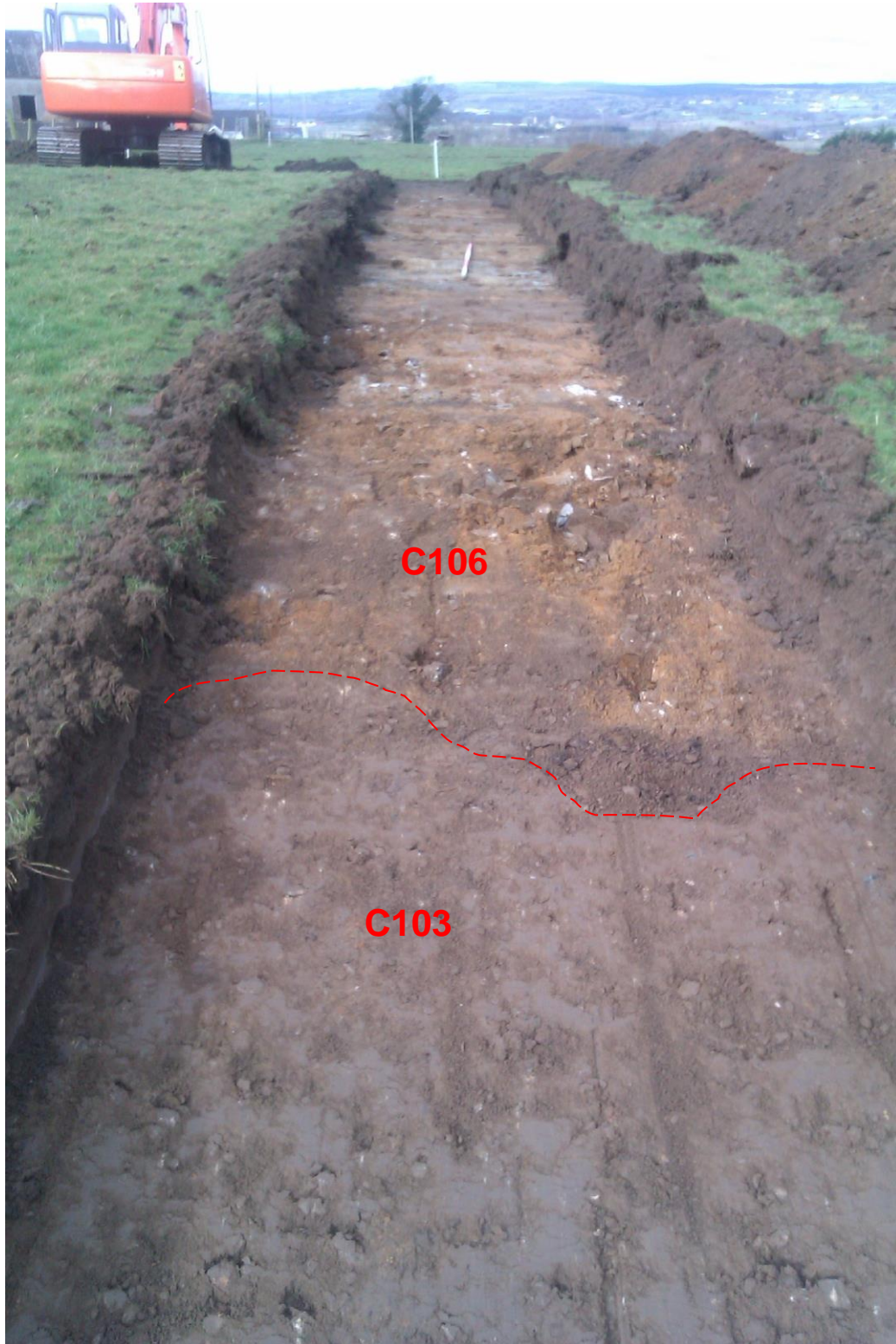
Plate 5: Trench 1 during evaluation showing brown sandy clay at south-eastern end, looking north-west
