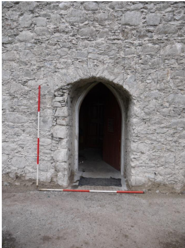
Plate 5: Entrance showing alterations made to the left hand side
