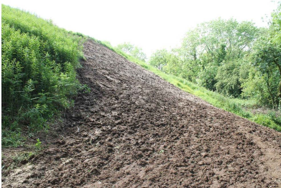
Plate 6: The slipped area following consolidation, looking west. Grass seed was spread on top of the exposed soil to aid in the consolidation of the monument.
