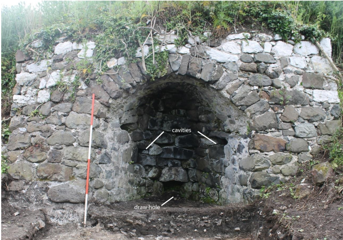
Figure 14: Cavities and draw hole within the arched recess, looking west.
