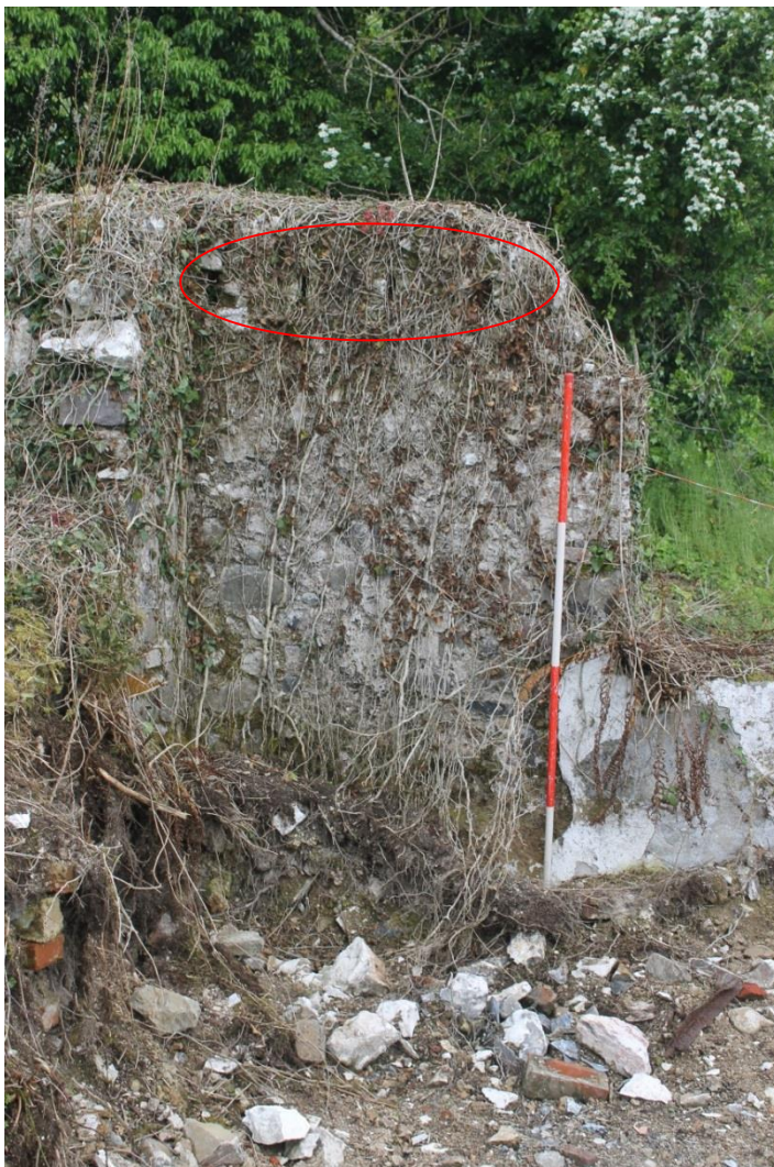
Figure 11: First floor joist holes in the NW corner of the second room, circled in red.
