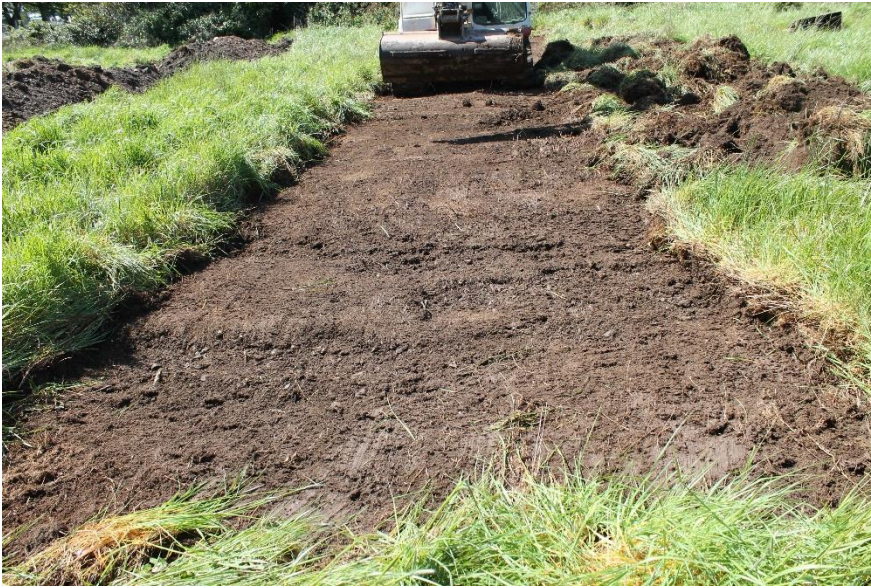
Figure 15: Trench 3 following removal of sod layer C301, looking southwest across topsoil layer C302.
