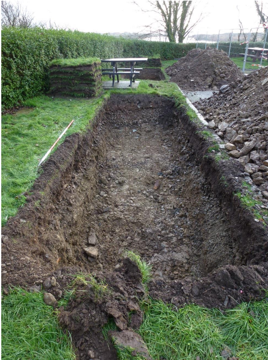
Figure 10: Trench 3A following partial excavation of redeposited boulder clay (307), looking southeast. For health and safety reasons excavation was halted after this photograph was taken. Scale 2.0 metres.
