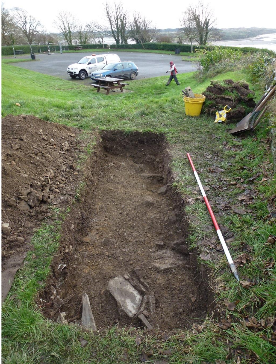
Figure 4: Trench 1A following excavation of the probable demolition deposit of mortar fragments and stone in a greyish brown silty clay loam soil matrix (104), exposing the truncated surface (105) of the probable slab-lined drain (108) and possible cut feature or natural hollow (110) within the surface of the redeposited or in situ mineral subsoil (111), looking northeast. Scale 2.0 metres.
