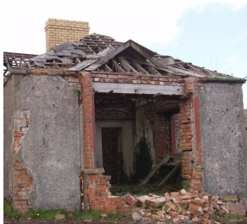
Pl 4 Remains of canted bay window before being blocked up (NT Photographic Collection)
