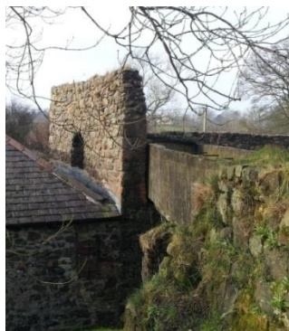
Fig 6. View of South wall of the Corn Mill with arched window – - the flume is seen passing through the building. (GT –I1900, 1)
