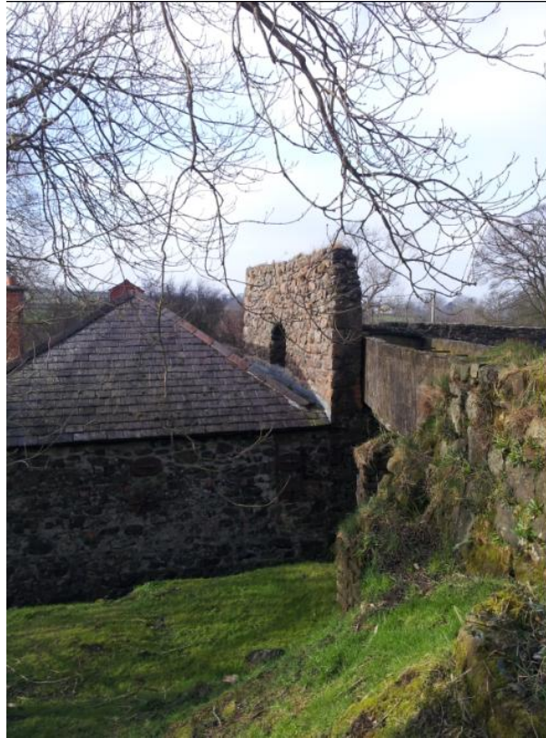
Fig 10. Single story roofed Paper Mill Machine Room facing east with remains of south wall of Rag Store and Engine Room (GT-I1900, 2 )
